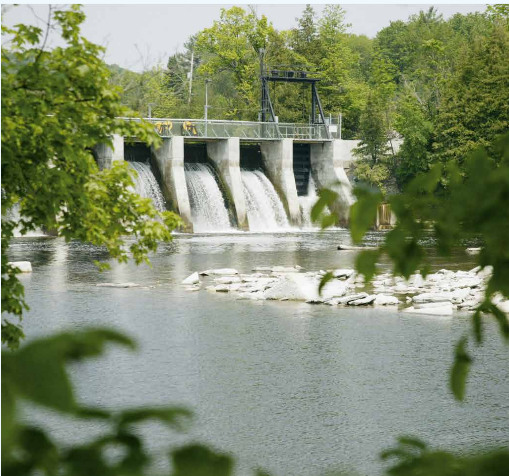
Glen Miller, an 8 MW run-of-river hydroelectric facility on the Trent River near Trenton.
