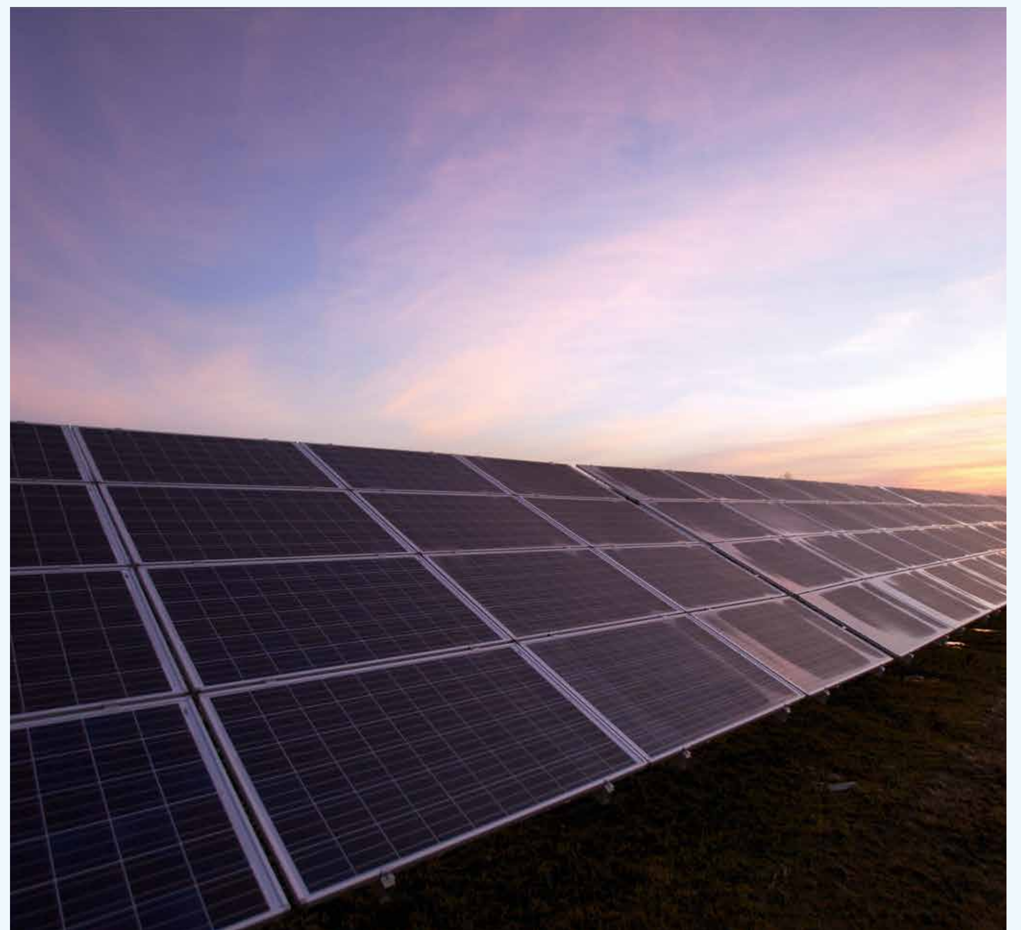
Stardale, a 27 MW solar photovoltaic facility in St. Eugene near Hawkesbury.
