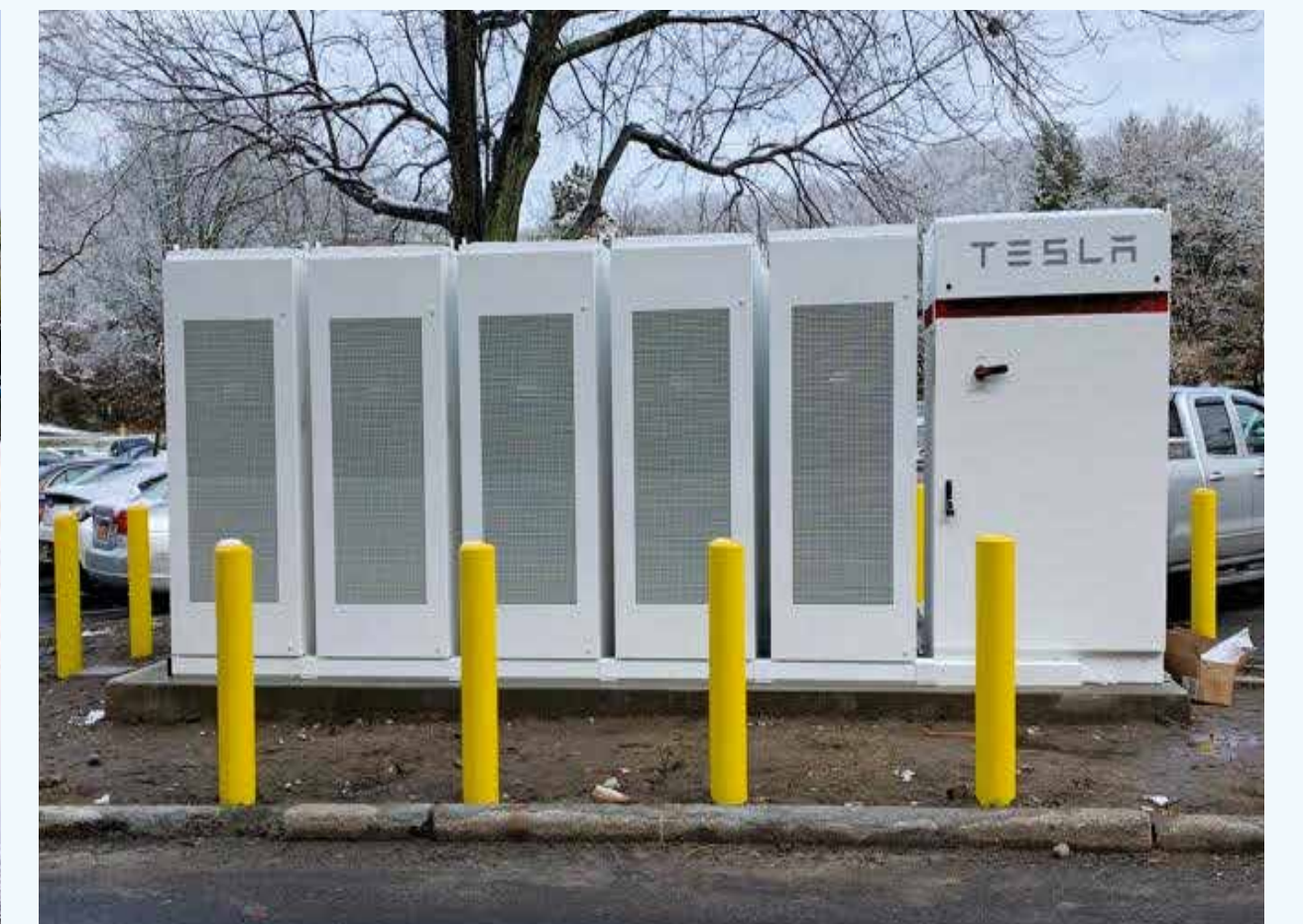
ENERGY STORAGE 5 MW
